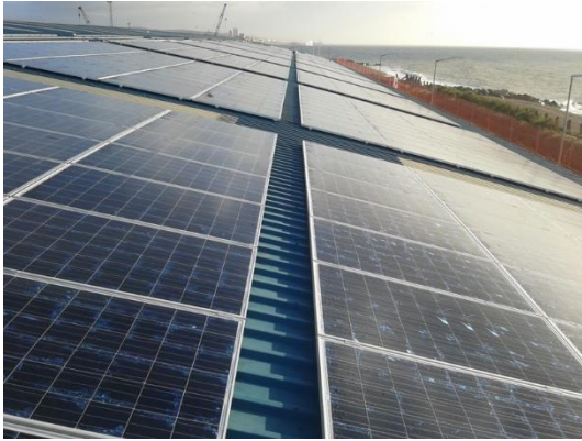
Solar panels on warehouse roofs
